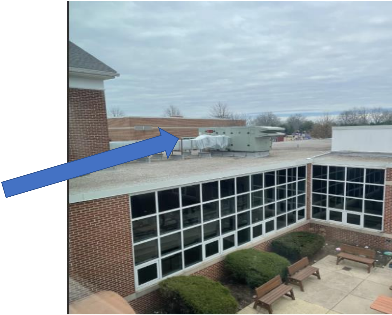
A new HVAC (Heating, Ventilation, and Air Conditioning) system has been installed.
